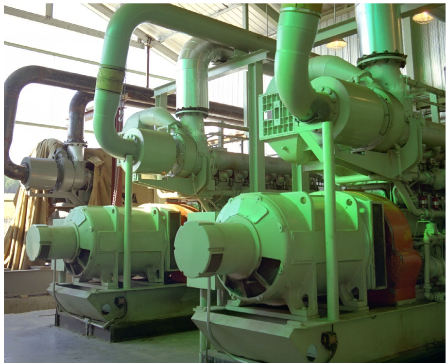
Heat exchangers, distillation columns and compressors are predominant applications of predictive maintenance.
